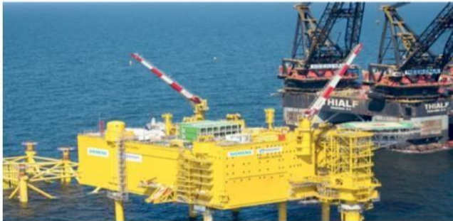
Figure 3: HelWin2 offshore HVDC platform of Siemens
